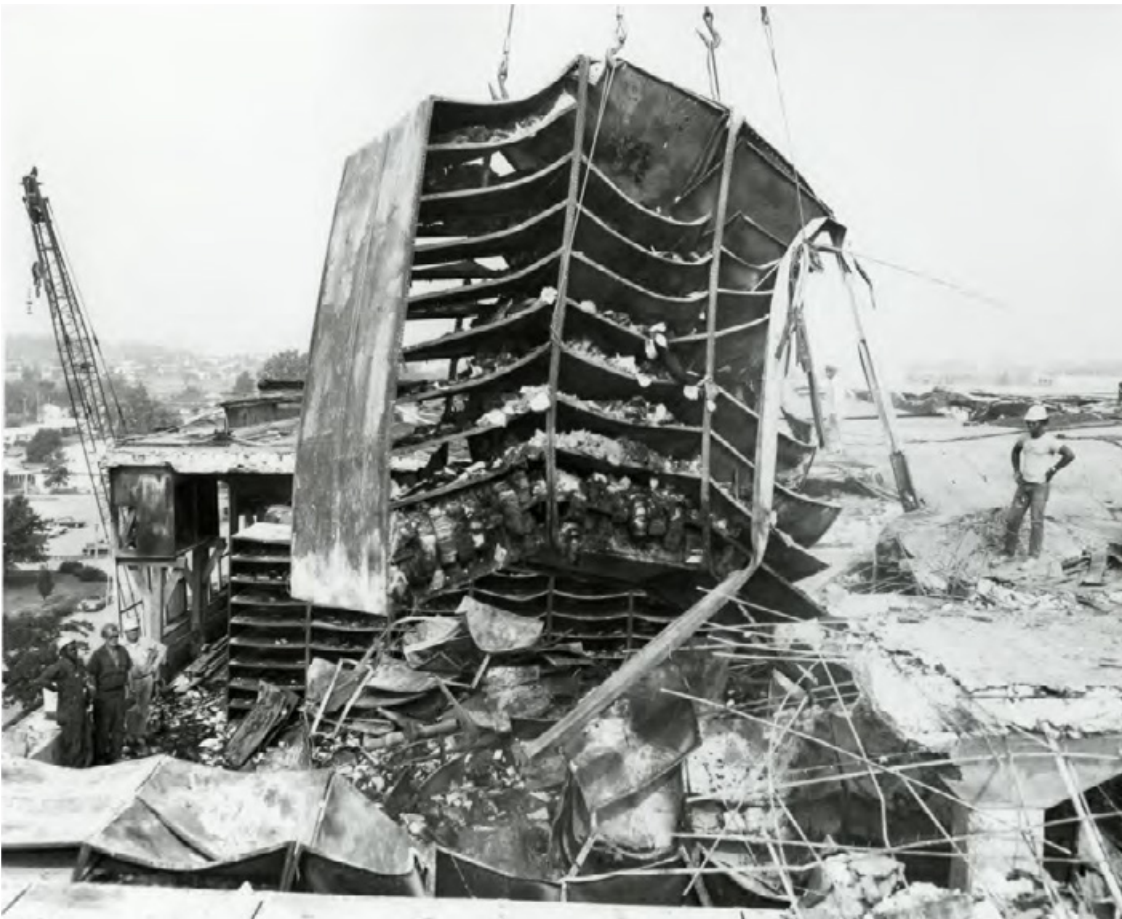
FIGURE 1. Aftermath of the 1973 fire at the National Archives, Military Personnel Records facility, in St. Louis, Missouri. Photo shows shelving being pulled from the damaged building. This disastrous fire destroyed approximately 16-18 million Official Military Personnel Files. There were no duplicate copies, no microfilm copies, and no indexes created prior to the fire. - Prologue , July 16, 2013 and NARA website
